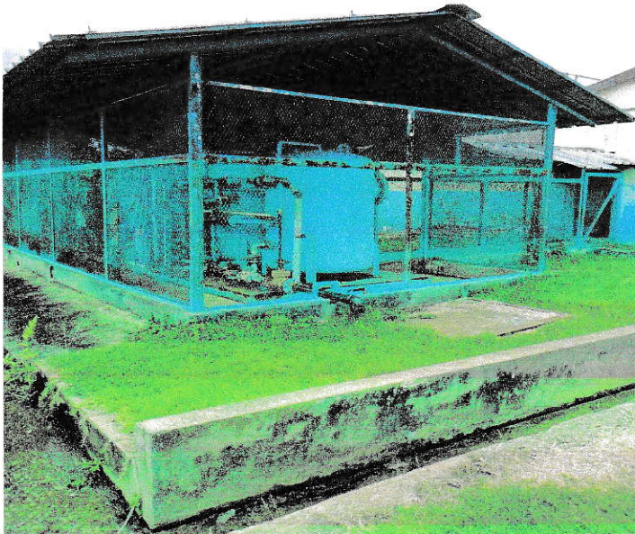
Station eau potable Okondja
