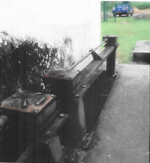
Station Assango: Batardeau hors service
