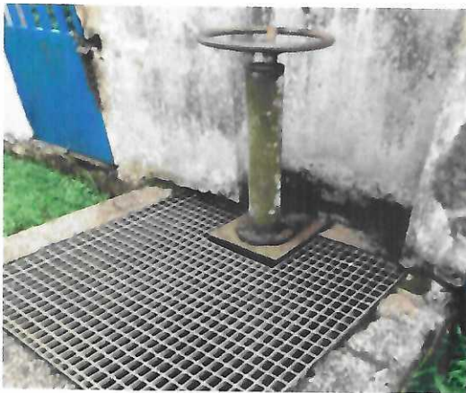
Station Meba: Batardeau hors service
