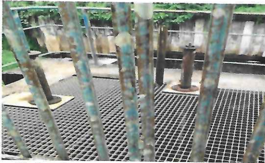
Station Saza: Batardeaux hors service
